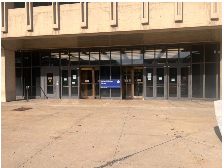
Image Description: Six entrances in total, two sets of doors on either side of two revolving doors. The door furthest to the right is the accessible door with the accessible push button. The concrete ground is textured and cracked.
