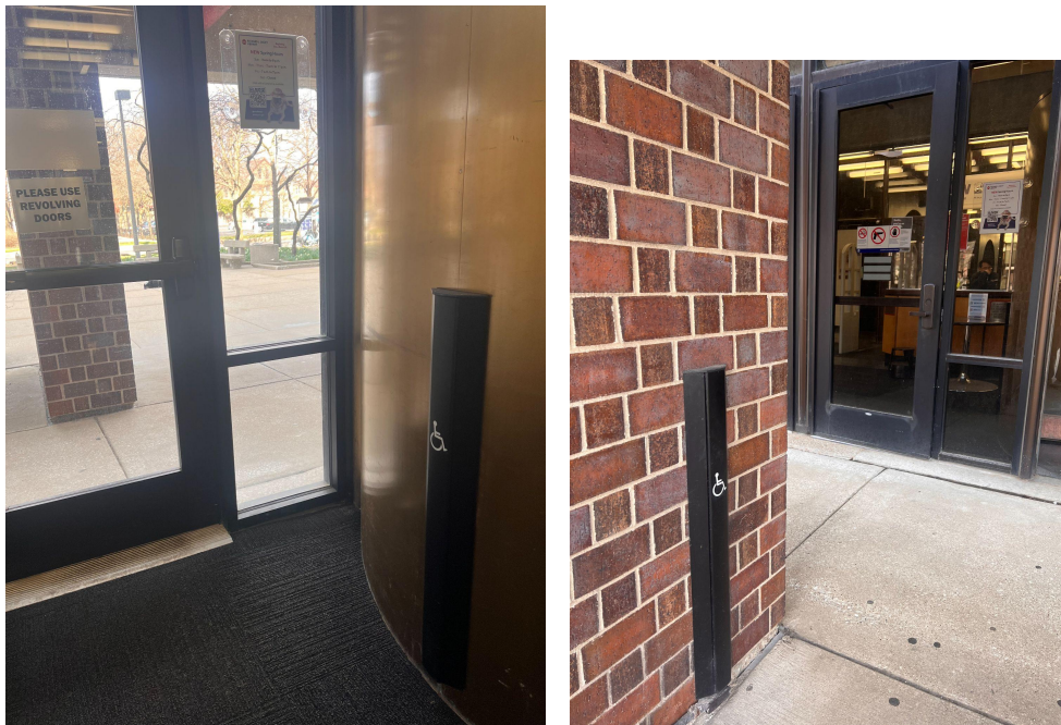
Image Description: (Left) A closed accessible door with an accessible push button propped onto a wall to the right of the image. (Right) A closed accessible door accompanied by an accessible push bar located to the left of the screen onto a brick wall.
