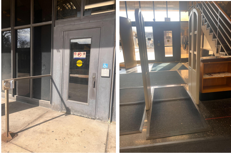
Image Description: (Left) Accessibility door accompanied by an accessibility button elevated to the left of the image. (Right) 2 paralleled metal detectors standing five feet away from the accessible entrance to the library. Carpeted floor is not leveled with a bump between the two standing detectors.
